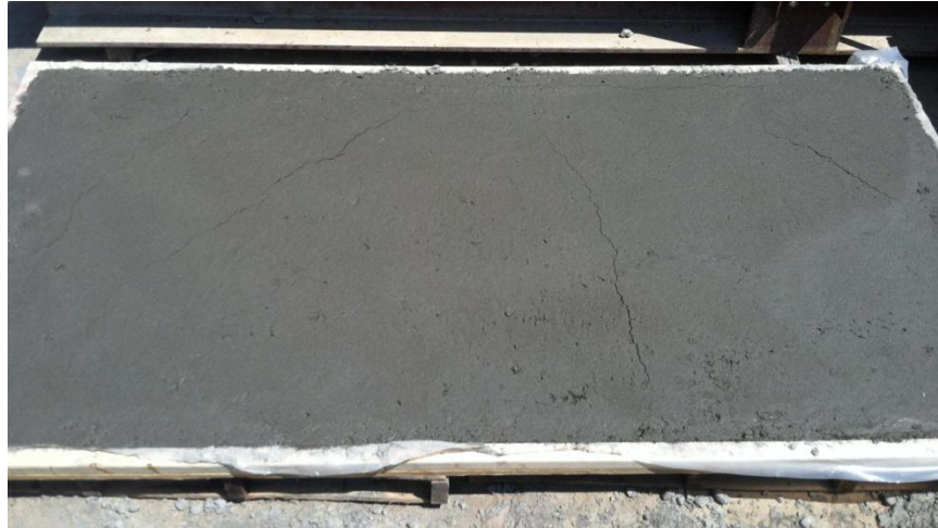
Figure 4.13 Slab After Formation of Plastic Shrinkage Cracks
