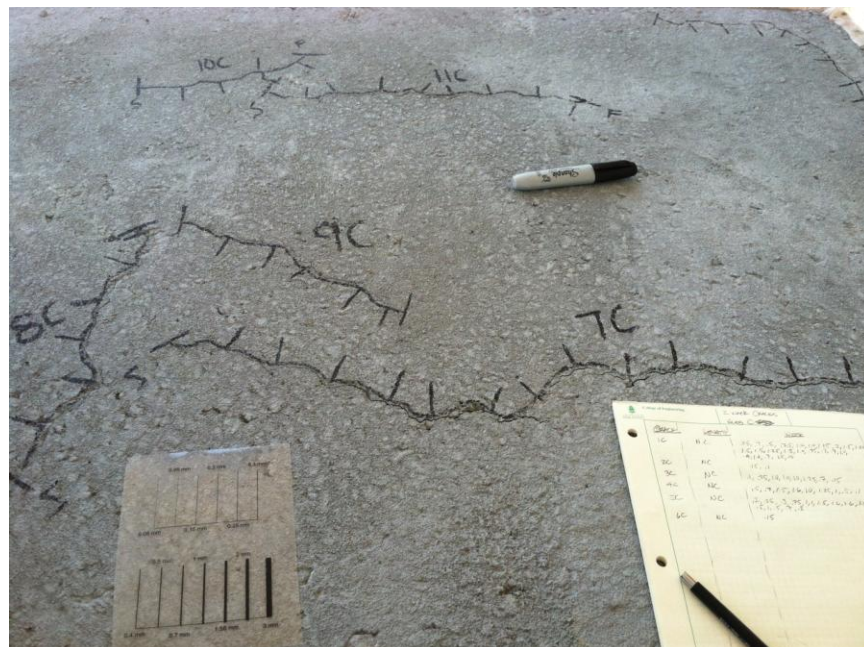
Figure 3.13 Test Slab During Crack Measurements
